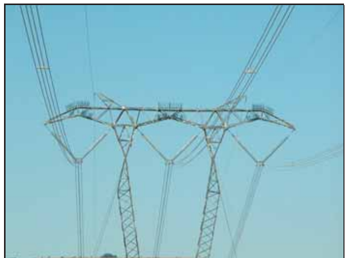
Figure 6: Plastic “Bird Guards” are placed on transmission towers to prevent birds from perching in critical areas (above conductors)
