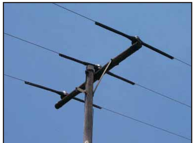
Figure 3: “Raptor Protectors” are used to insulate the conductors one meter either side of the cross arm on wooden T-pole structures.
