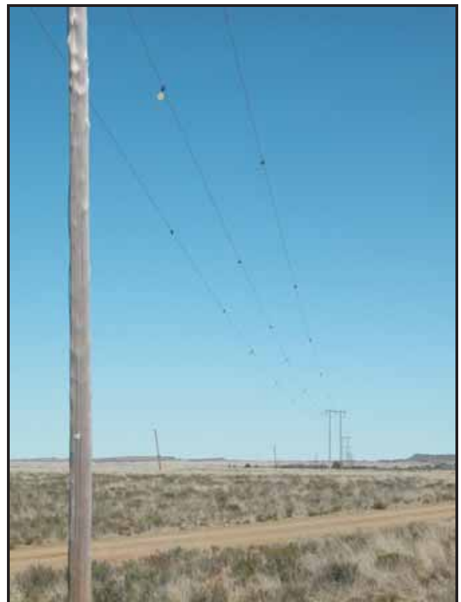
Figure 5: “Bird Flappers” are fitted onto the overhead conductors at ten meter intervals to make the conductors more visible.
