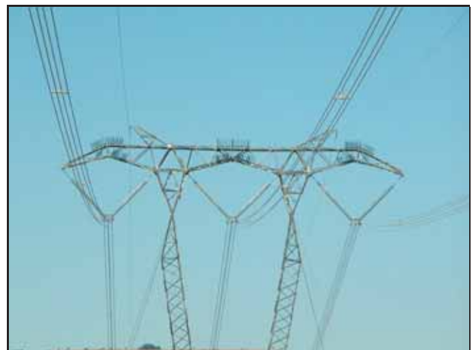
Figure 6: Plastic “Bird Guards” are placed on transmission towers to prevent birds from perching in critical areas (above conductors)
